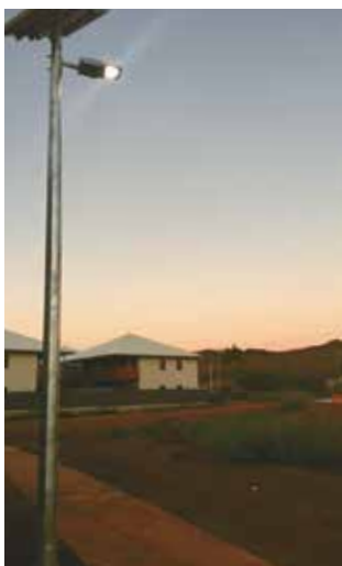
Solar footpath lighting
