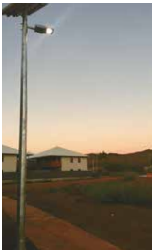
Solar footpath lighting
